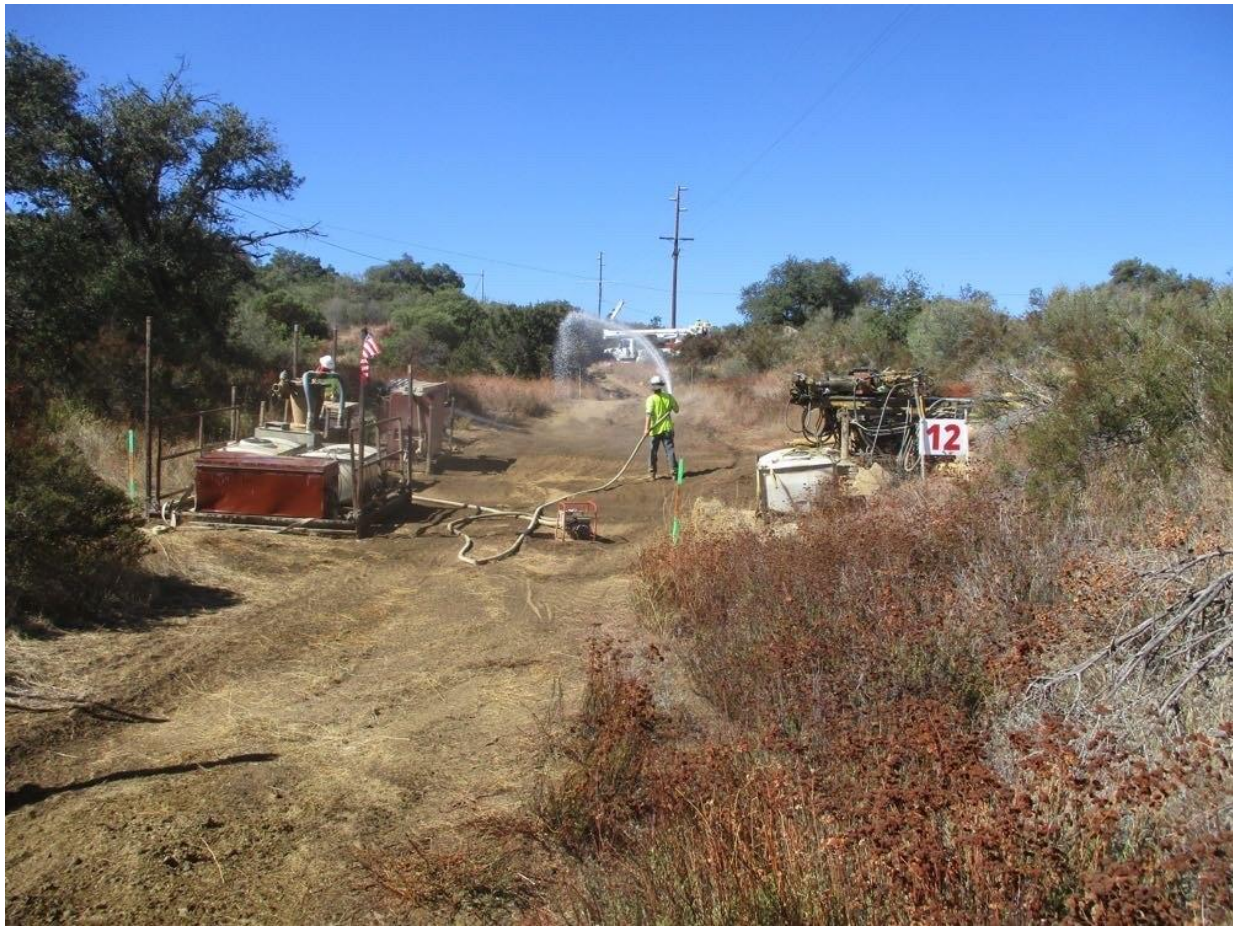
Photo 1: In preparation for the removal of micropile drilling equipment via helicopter external load operations at Pole Z172744 (TL 629A), the area was observed being watered down to mitigate dust emissions anticipated from rotor wash in accordance with APM AIR-02, APM AIR-05, the Aviation Safety Plan, and MM PHS-5.
