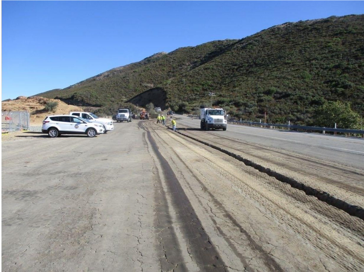
Photo 6: During preparation for paving over the underground distribution line trench at C 440 Phase 1, a street sweeper was observed being operated along Sunrise Highway to clean the road and prevent off-site erosion in accordance with the Erosion Control Plan and SWPPP.
