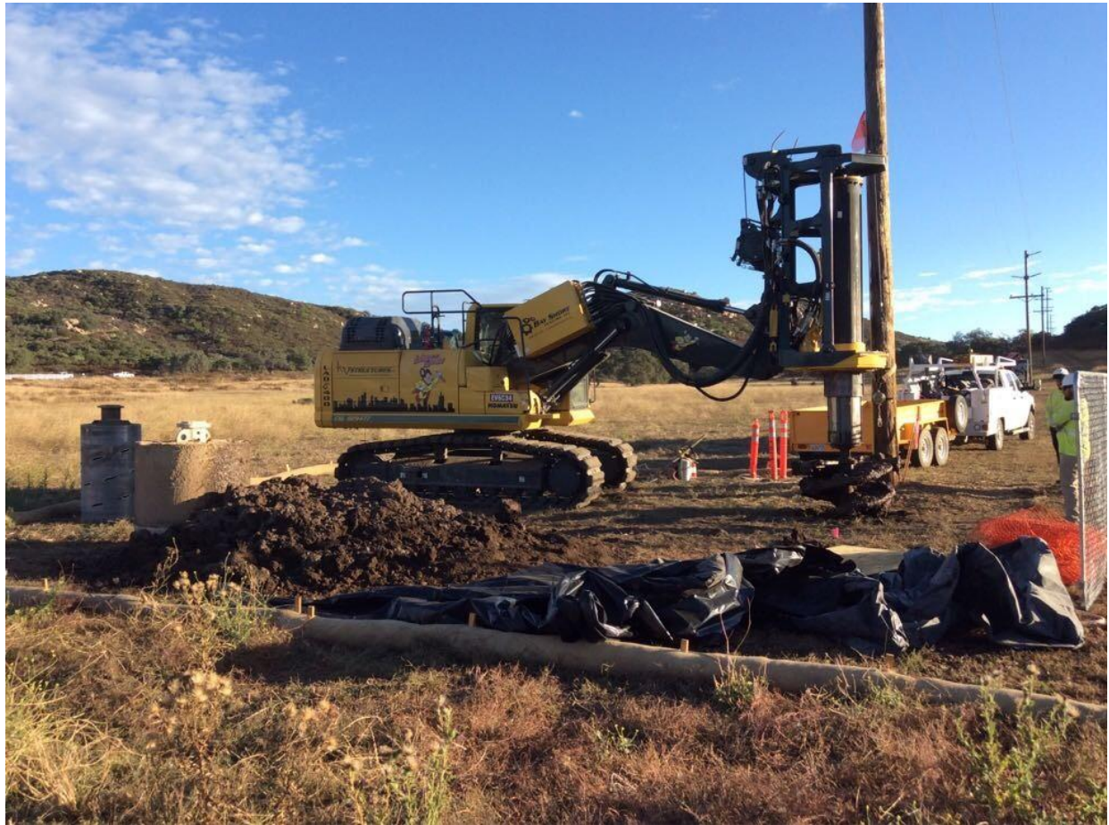
Photo 5: To prevent off-site erosion during pole hole drilling at Pole Z272949 (TL 625C), the drill operator placed dirt spoils within the designated workspace surrounded by fiber rolls in accordance with the ECP (MM HYD-1) and SWPPP (MM BIO-7).
