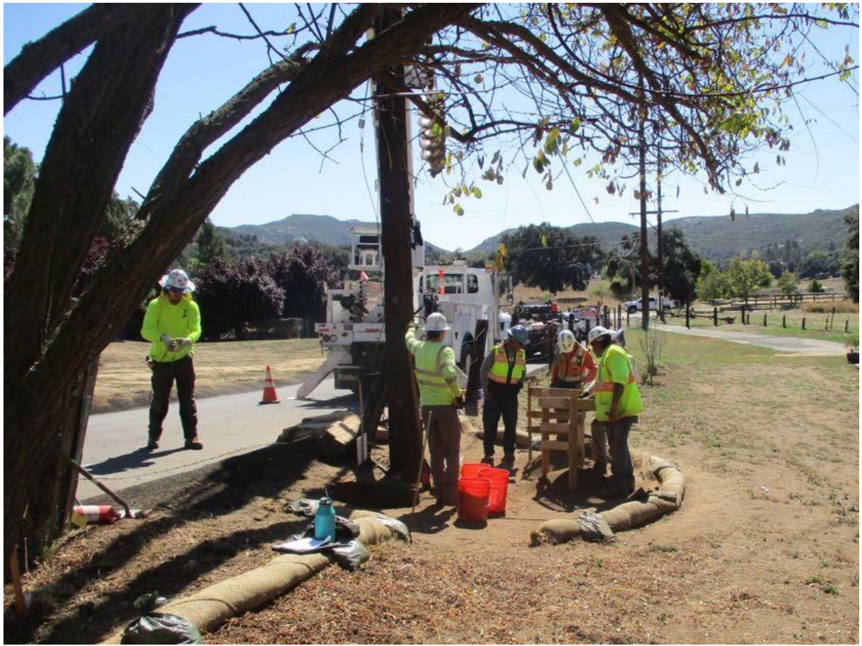
Photo 2: Cultural monitors were observed leading an excavation of both the pole hole and the trench used for ground wire and rod installation at a site along TL 629A, and screening excavated material for potential cultural resources in accordance with the Historic Properties Management Plan, MM CUL-1, and APM-CUL-04.
